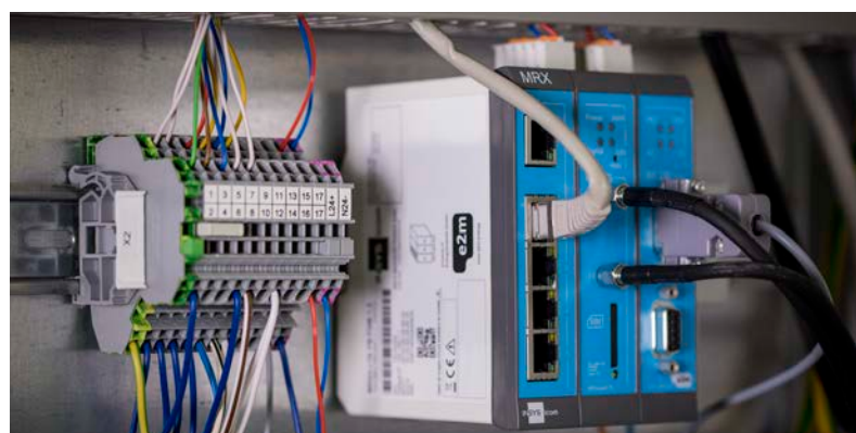
Gateway of the Virtual Power Plant © ahnenenkel.com/Silke Reents
